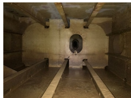
Gambar 7: Water Ballast Tank .
