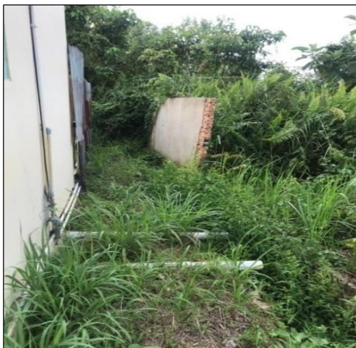
Figure 7. One of the documentation of building damage due to land subsidence
