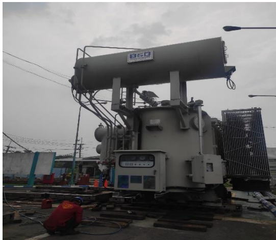
Fig. 2. Transformer 60 MVA at Surabaya Barat Substation
